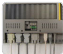
Downward I/O cabling
